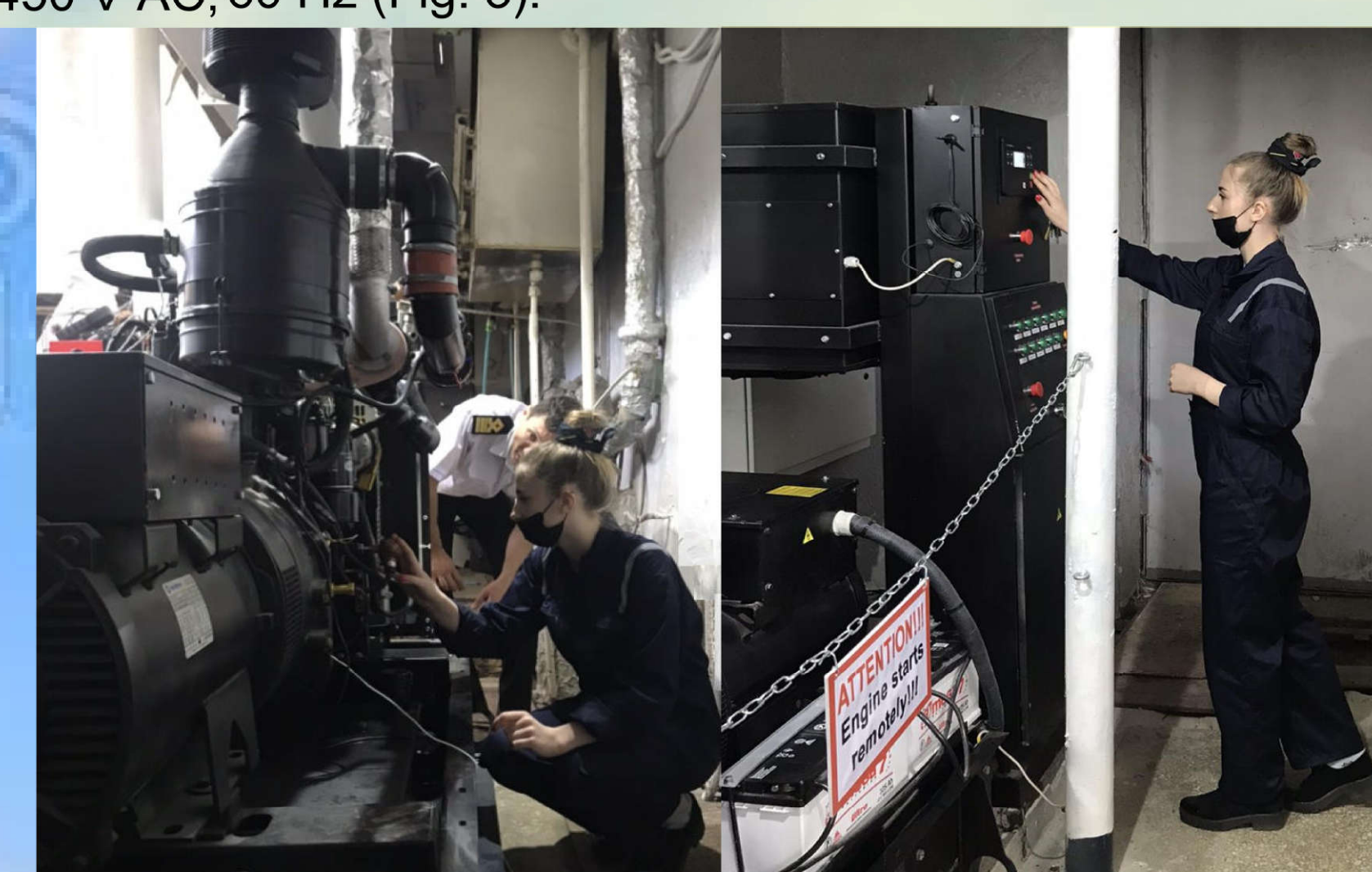
Figure 3. Participant in the real conditions preparing to start and start emergency diesel generator in the academic engine room laboratory
